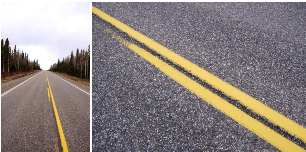
Figure 1. Representative images for Highway 11 condition west of Cochrane.
